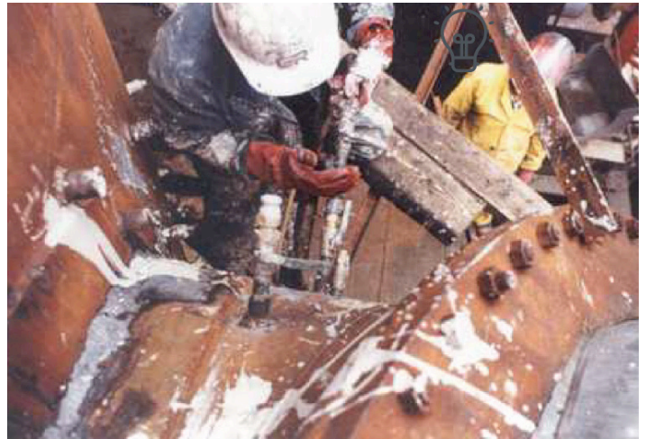
7. Note two on/off valves. First valve closest to tower is open. Second valve on line is closed. Now ready to start pressure grouting.
